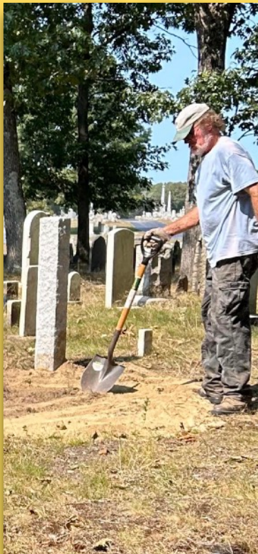
Thank you to Mark for helping to install the new granite posts.
