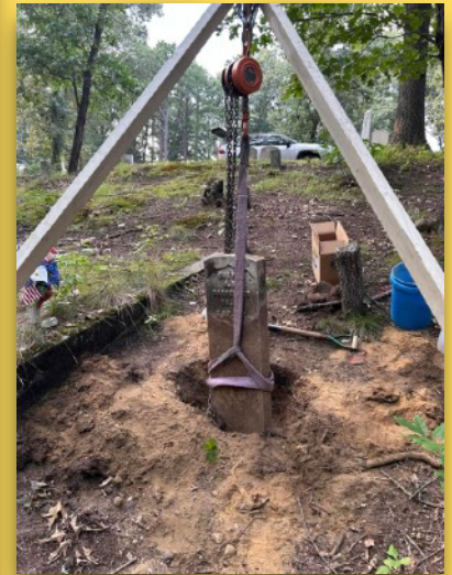
The last veterans headstone has been raised and re-set. All together, 27 veterans stones have been cleaned, re-set and are now finished. Now work has shifted to restoring fences and planting flowers.
