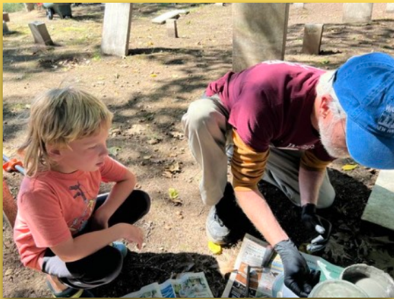
Mark Laprade has an interested audience as he prepares epoxy for a repair. Gayle's grandson, Miles, is our youngest volunteer!
